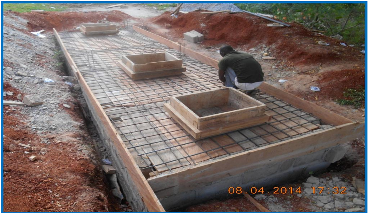
Figure 4: Ongoing construction of Anaerobic Baffled Bio-Digester showing steel reinforcement of top slab
